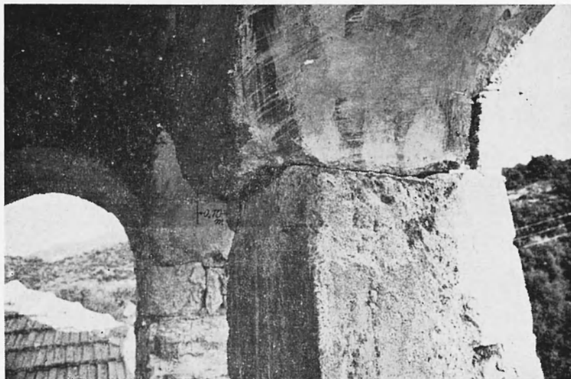
Fig. 29. Construction joint with no connection of the two adjacent parts, caused a dislocation of the top part of the church steeple at Kaloudi.
