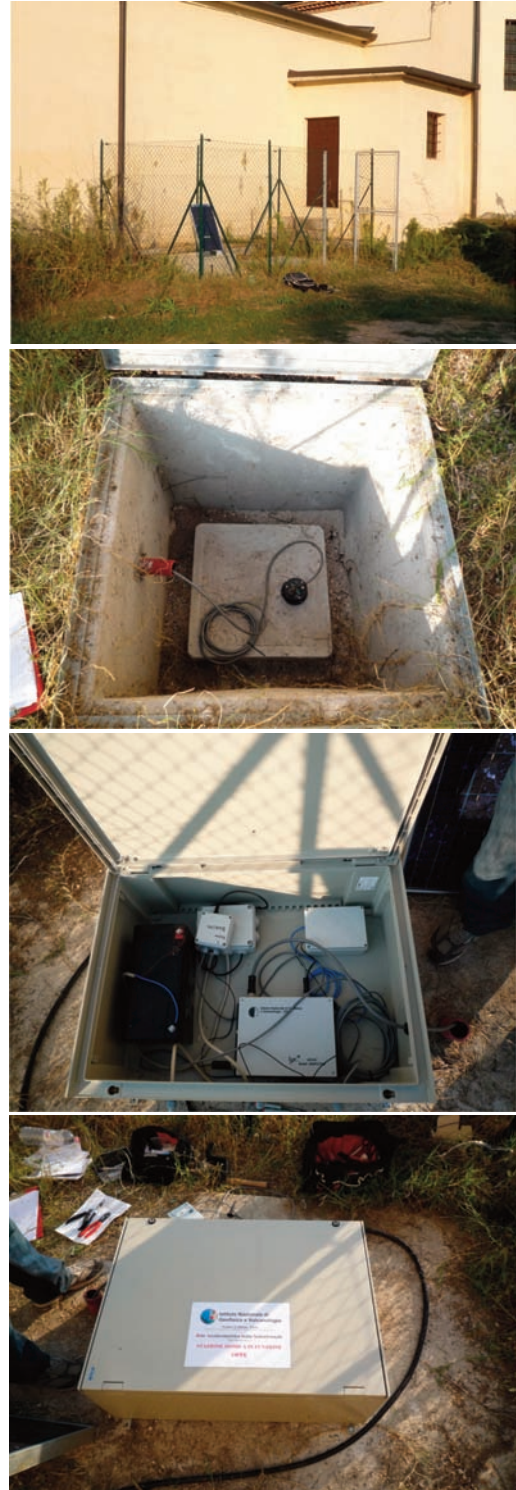
Figure 5. Typical installation arrangements. From top to bottom: external view; concrete basement where strong-motion sensor is anchored; plastic box that includes the recording system (open); plastic box (closed).
