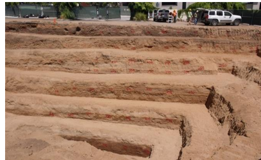
Figure 4b: Photograph showing a portion of the 9+ m deep trench excavated in the parking lot of the Tower Records building, which is also the East Millennium site. The footprint of the trenches is shown in light turquoise on the figure to the left. A demonstrably not active fault with about 50 cm of total displacement was exposed near the bottom of the trench. Photo courtesy of Group Delta Consultants.
