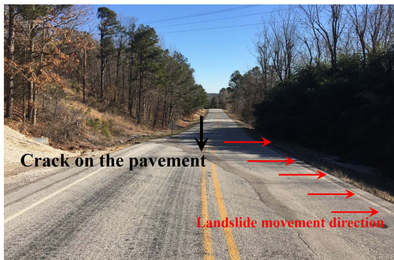
Figure 1. A sample longitudinal crack observed on the pavement.
