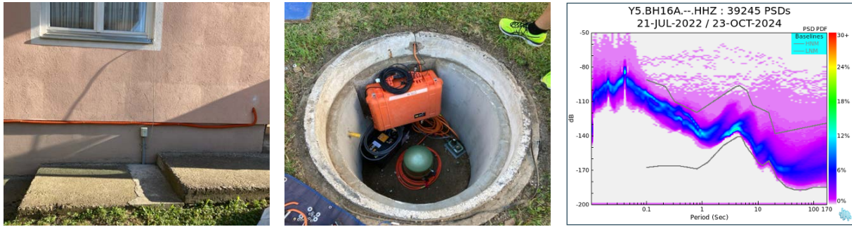
Figure A16. BH16A, Dobož, is installed in an urban open field in the backyard of the local meteorological observatory Dobož. The sensor is inside a seismic vault on a concrete base at the edge of a dense urban village.
