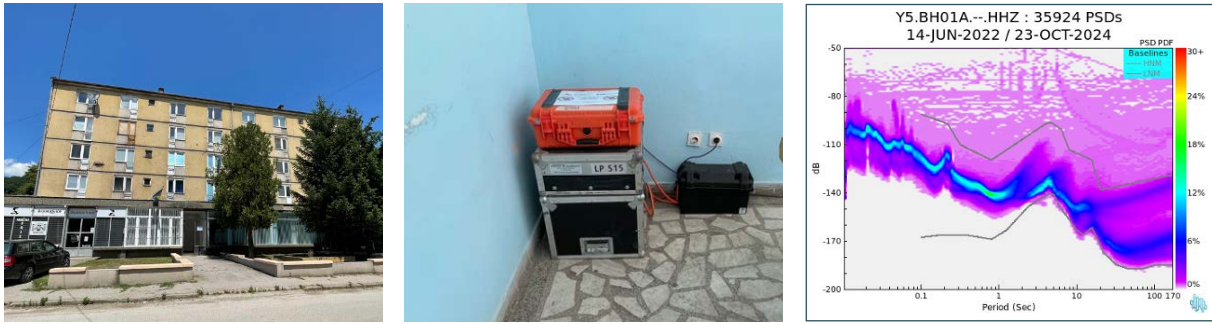
Figure A1. BH01A, Vitkovići, Gorazde, is installed in a municipal building on the ground floor, in the central southern part of the building, which is used only for monthly meetings. The sensor is placed in the northeast corner of the room on floor tiles. The building is situated in a dense urban village.
