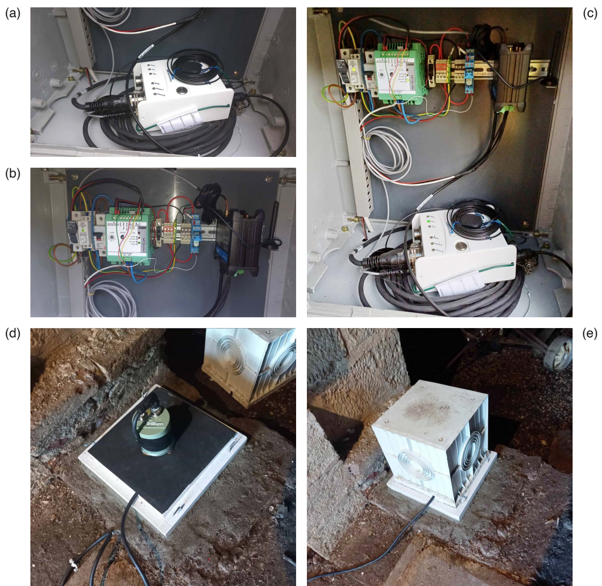
Figure 3. Components of an OGS seismic station for the AdriaArray project: (a) the Nanometrics Centaur acquisition system; (b) the mobile internet router with switches; (c) both integrated in a closed metal cabinet; (d) the Nanometrics Trillium Compact 120 sec broadband seismometer, installed on a marble plate; (e) the sensor covered with plastic thermal insulation.
