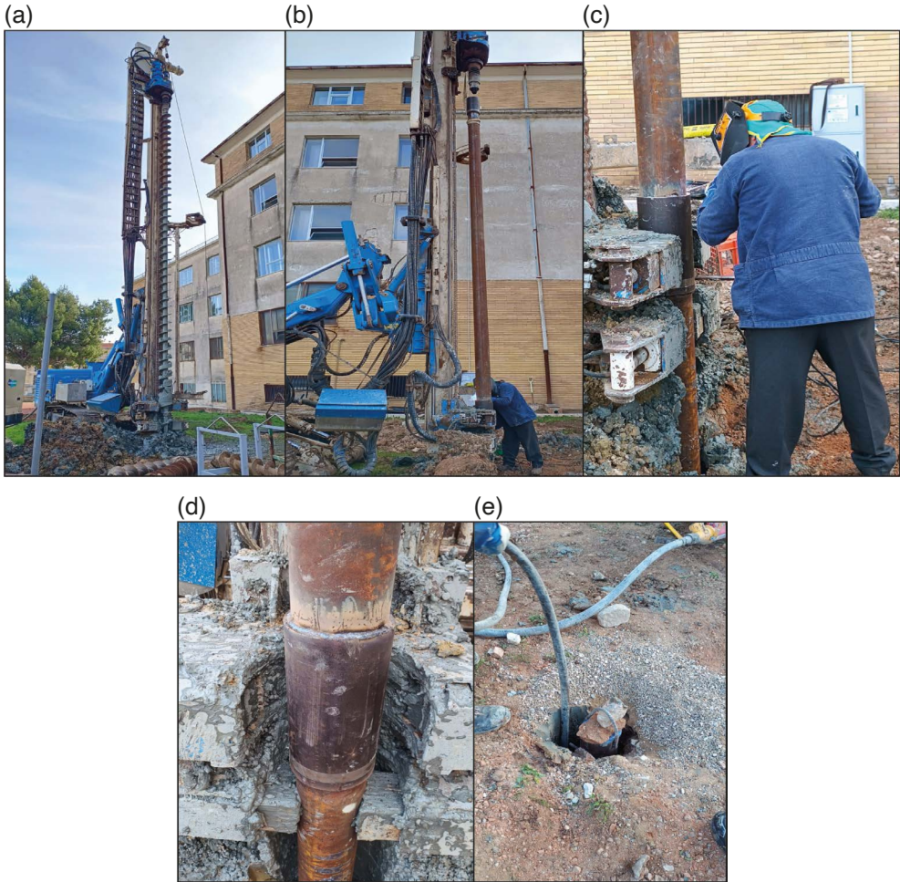
Figure 6. (a) Drilling operation of the well. (b) Phase of lifting and alignment of one of the steel pipe segments. (c-d) welding process to join two segments through the external steel joint and result. (e) Pouring liquid cement into the space between rocks and the external side of the pipe.
