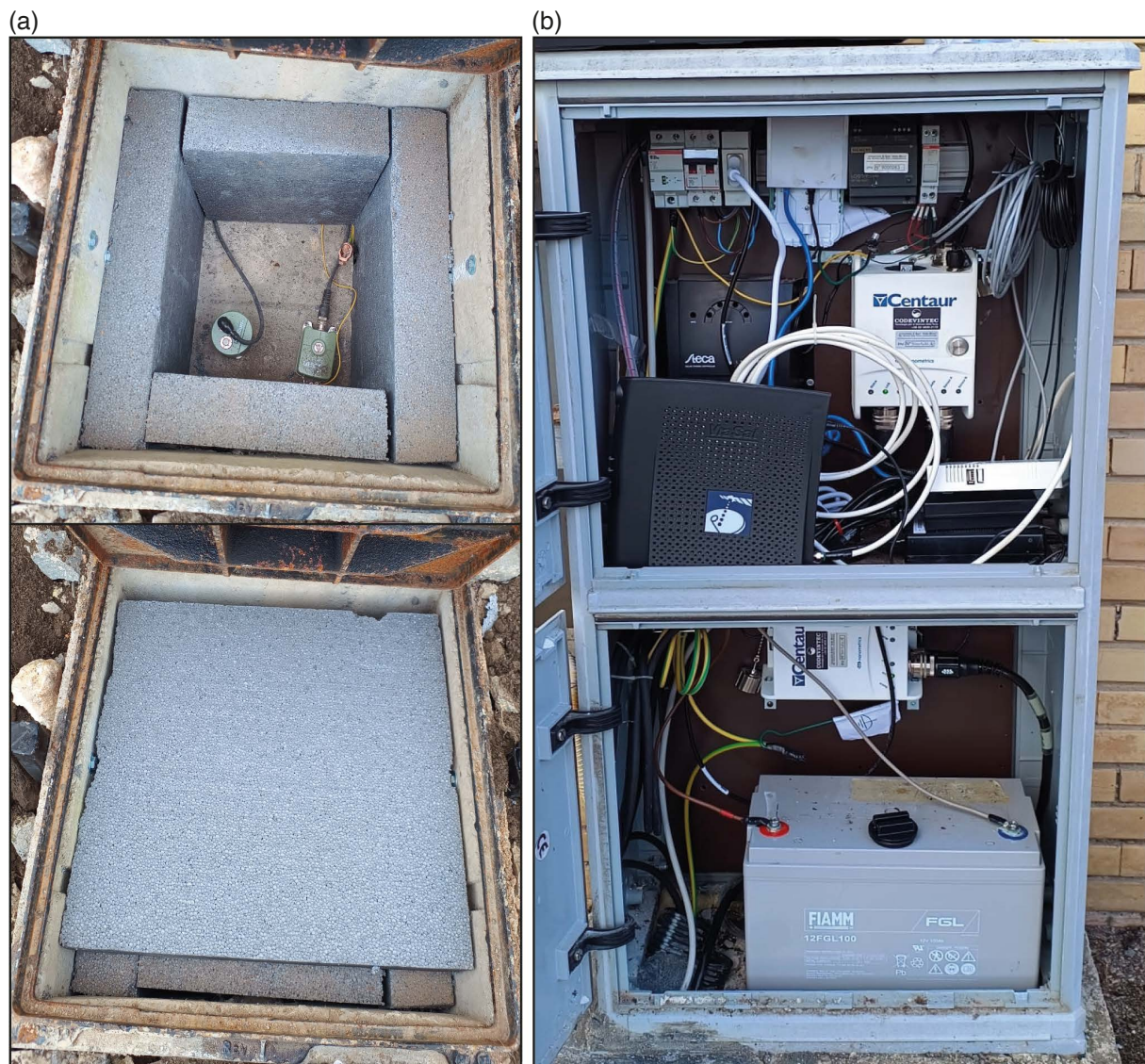
Figure 3. The seismic station OT11. (a) Concrete manhole with thermo-insulating cover in polystyrene. (b) Plastic cabin containing data loggers.
