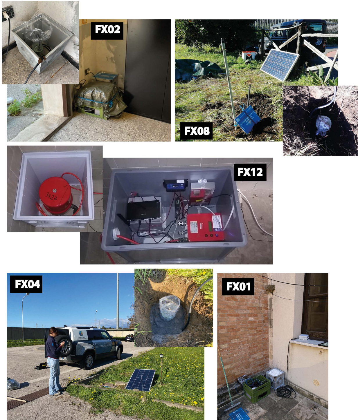
Figure 3. Examples of station installations at representative sites.
