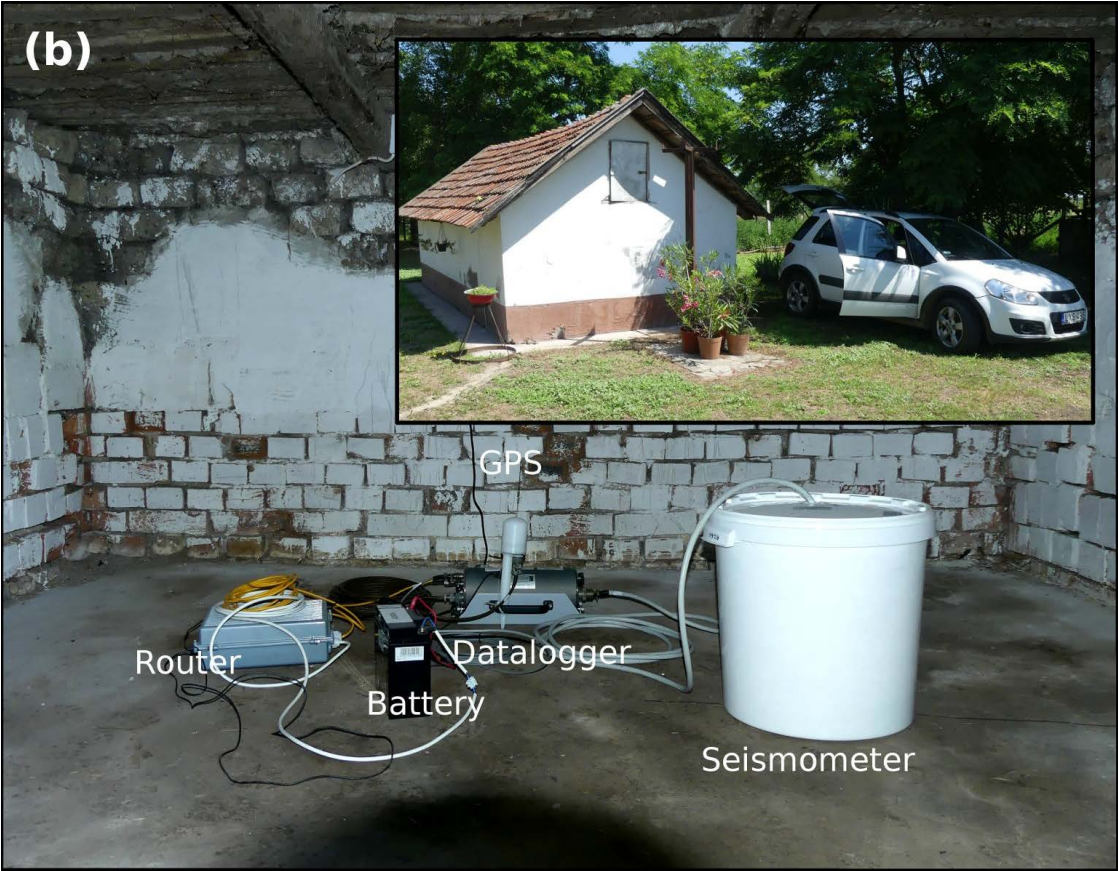
Figure 3. Two examples of installed temporary stations. (a) HU01A is installed in a cellar, the seismometer is placed on a granite slab, covered by a bucket filled with polystyrene packing foam peanuts. (b) HU06A sensor was placed on the concrete floor of an unused building.
