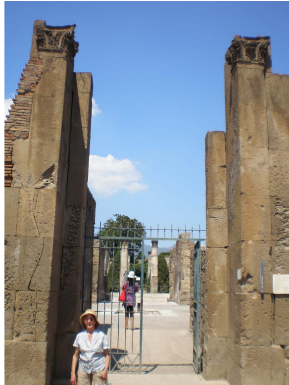
Figure 9. Cracks in the entrance portal of the House of Pansa (VI,6,1). On the left, below the capital, a brick support, built after the time of the excavation, is visible. The missing blocks may be those that fell into the street, shown by W. Gell in his 1921 Pompeiana guide.
