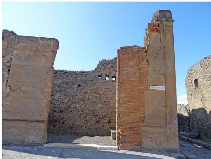
Figure 12. The pillars of the shop at the corner of Via della Fortuna and Vicolo del Labirinto (VI,12,6) show repairs with brick supports, likely due to damage from the AD 62 earthquake, as well as fractures that may have occurred later. However, as shown in historical photographs, these are not attributable to the 1943 bombings.
